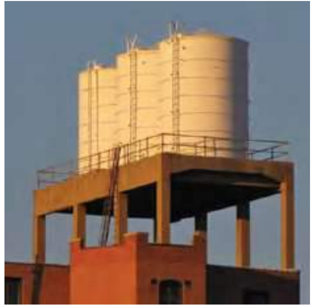
Overhead water tanks
